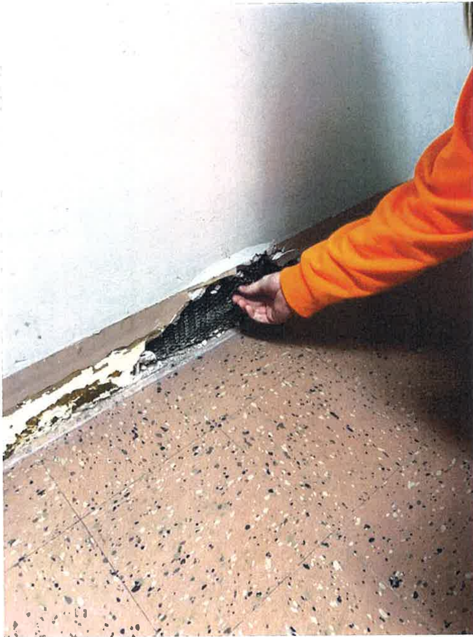
Sharp mesh wiring coming out from plaster where baseboard was removed
