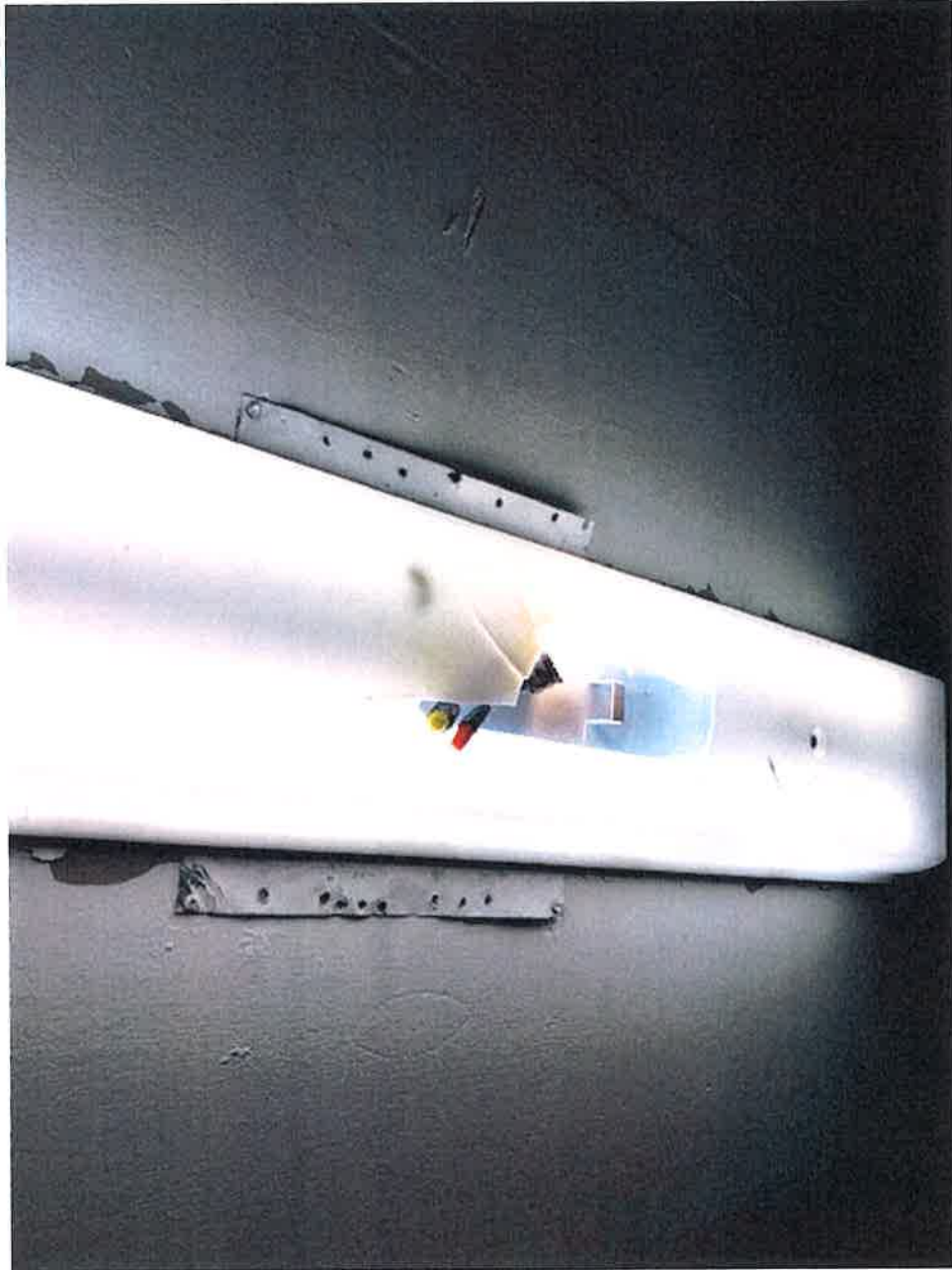
Broken light fixture in Sac Several Rooms had no lights at all or did not work
