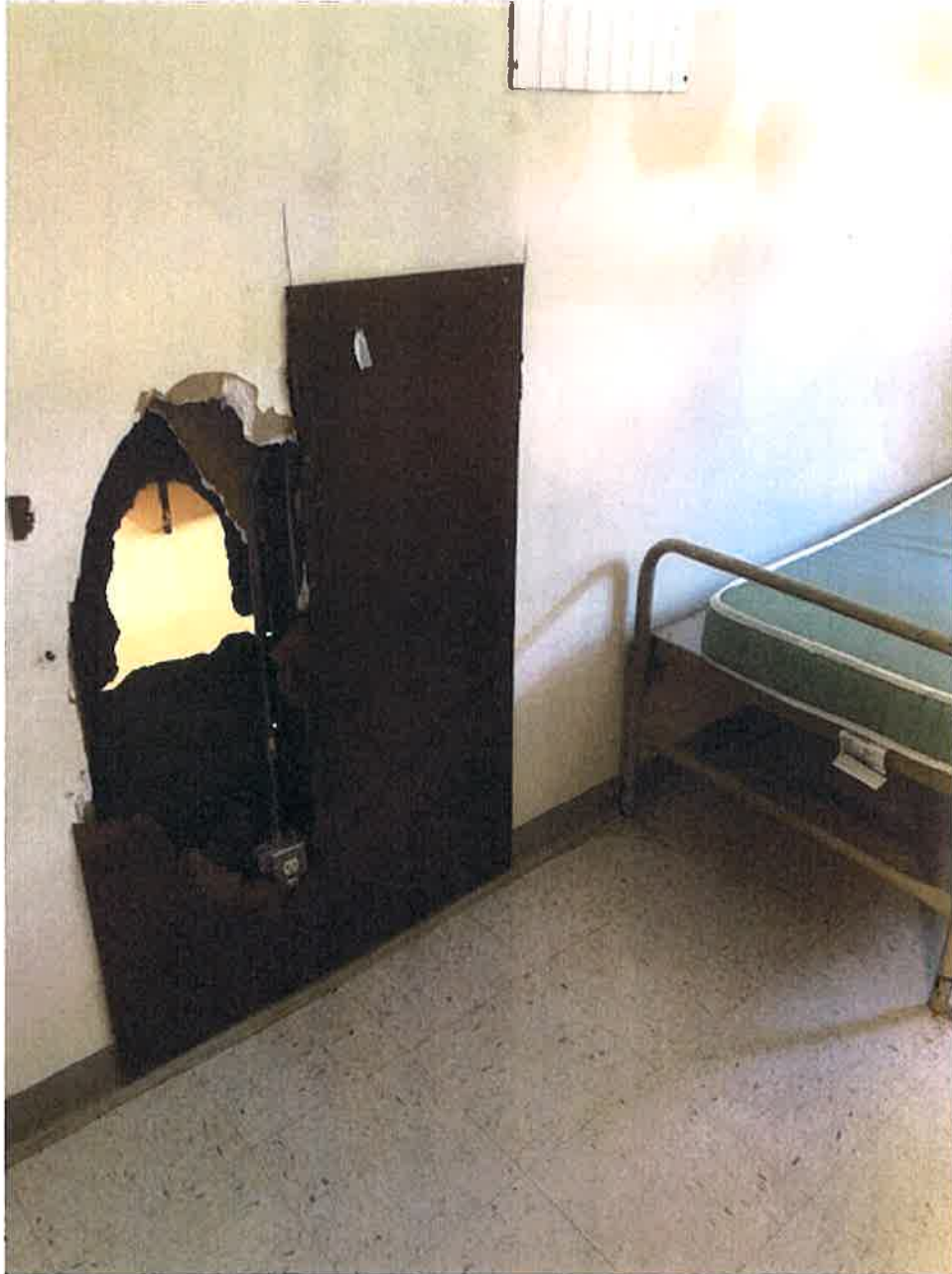
Holes in walls between rooms in Sac
