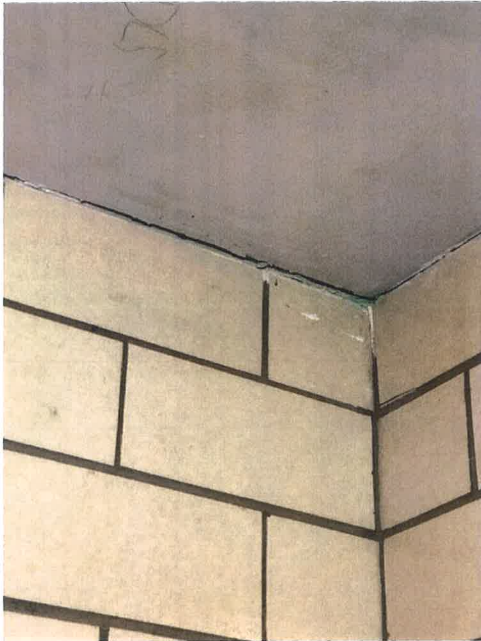
Mold in corner of an occupied room in Sac
