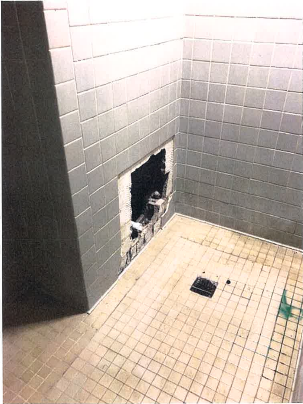
Sewer issue in LaFlesche
